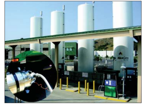
The East Valley fueling station in California, operated by the City of Los Angeles, has five LNG dispensers and three CNG dispensers. Photo courtesy of Chart Inc.
